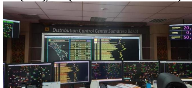
Figure 3. Ruang Distribution Control Center (DCC) UP2D SUMBAR
