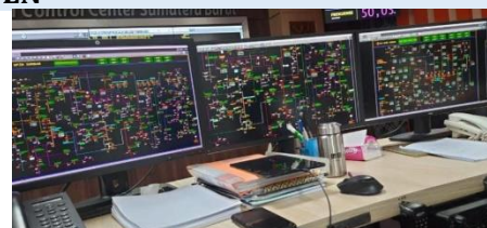
Figure 9. Tampilan Aplikasi SMART VU SCADA PLN UP2D SUMBAR
