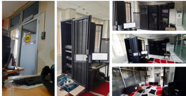
Figure 2. Server SCADA PLN UP2D SUMBAR
