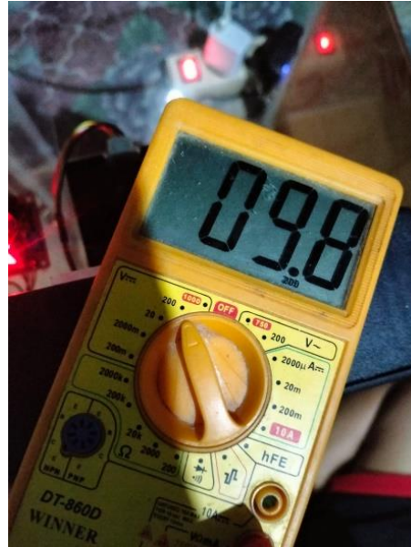
Figure 10: Motor Voltage Measurement When the Sluice Gate is Open
