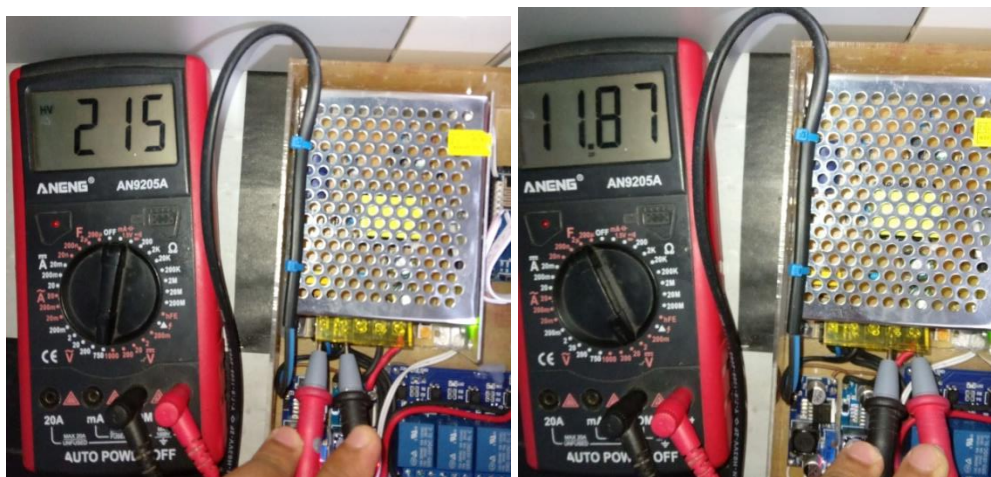
Gambar 6. Hasil pengukuran tegangan power supply
