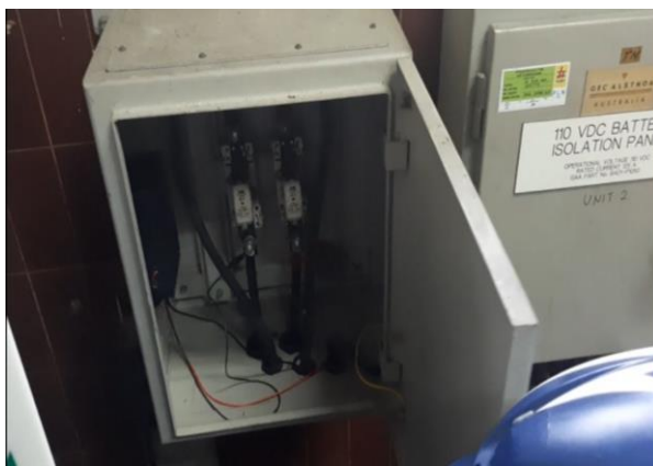
Gambar 6. Box panel monitoring baterai 110 VDC
